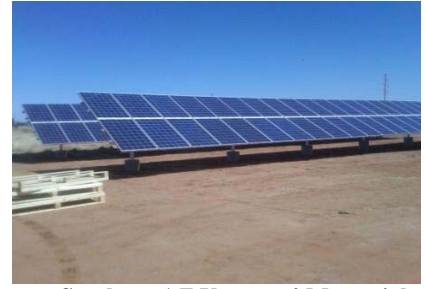
Southern AZ Veterans' Memorial Cemetery, Solar Photovoltaic Sierra Vista, AZ
