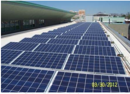
Solar Photovoltaic Arizona State Hospital, Phoenix, AZ
